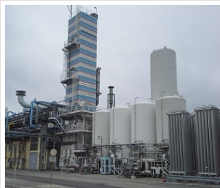
AlzChem air separation unit
