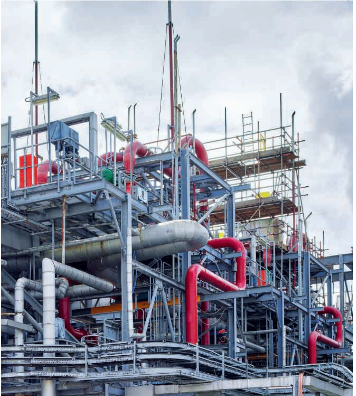
A boiler plant which can switch between operating on natural gas or hydrogen, depending on the availability of hydrogen from the cellroom
