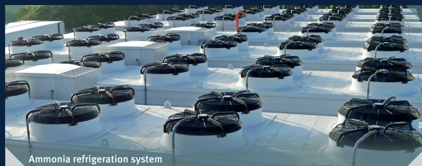
Ammonia refrigeration system
