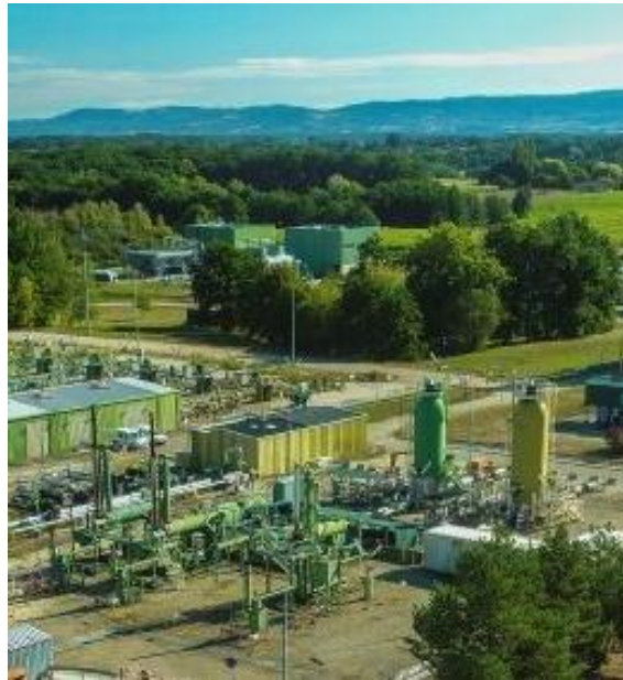
HypSTER, Ertrez France. 50 tonnes of hydrogen in EZ53 cavity will be followed by additional caverns to 6,700 tonnes.
