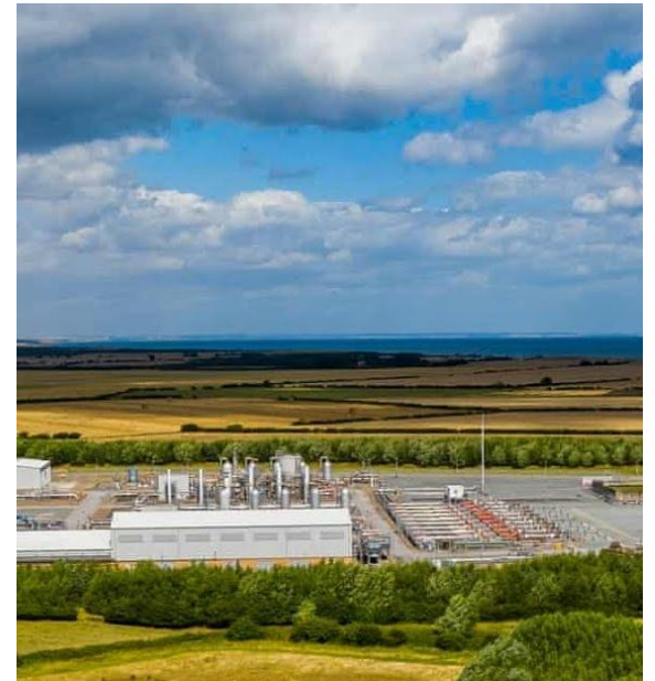
UHS to be implemented at an existing SSE site in Aldbrough on the Yorkshire coast in the UK.
