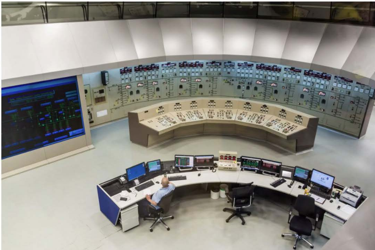
Itaipu dam control room - image courtesy of @sbh4 GmbH
