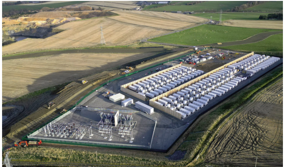
Huge utility-scale long-duration energy storage (LDES) facilities using lithium ion batteries are being implemented in many countries
